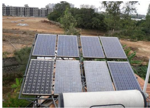
Picture 5 – Solar panels at the roof top
