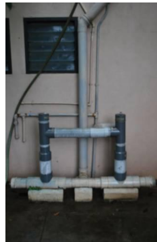
Picture 19 – Pop-up filter filtering the rain water before it goes to the sump.
