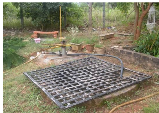
Picture 11 – Treated grey water going to the well which is then used to water plants.
